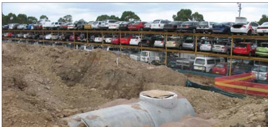
On-site detention pits at the Pickles Site
